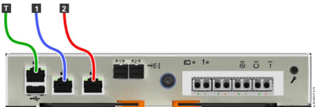
Figure 127. Connecting the Ethernet cables to a Storwize V5030 or Storwize V5030F system
